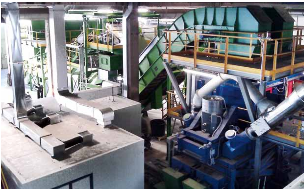
CarbonNext production plant with biostabilization
